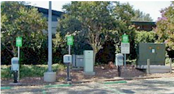
Figure 1. A typical pedestal-style charging station in a surface parking lot. Photo courtesy of ECOTALITY.
