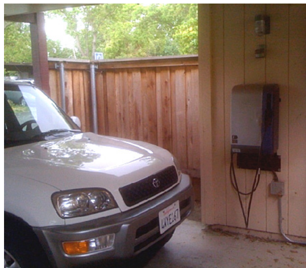
Figure 3: A wall-mounted Level 2 home charging station in a carport. Outdoor home charging stations can also be Level 1 and may not require covering. Photo courtesy of Plug In America.
